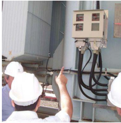
Figure 1 IEDs on the tank of transformer [1]
